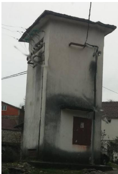
Slika 6.31. ZTS KOKORIĆI 1 PERVANI 10/0,4kV
